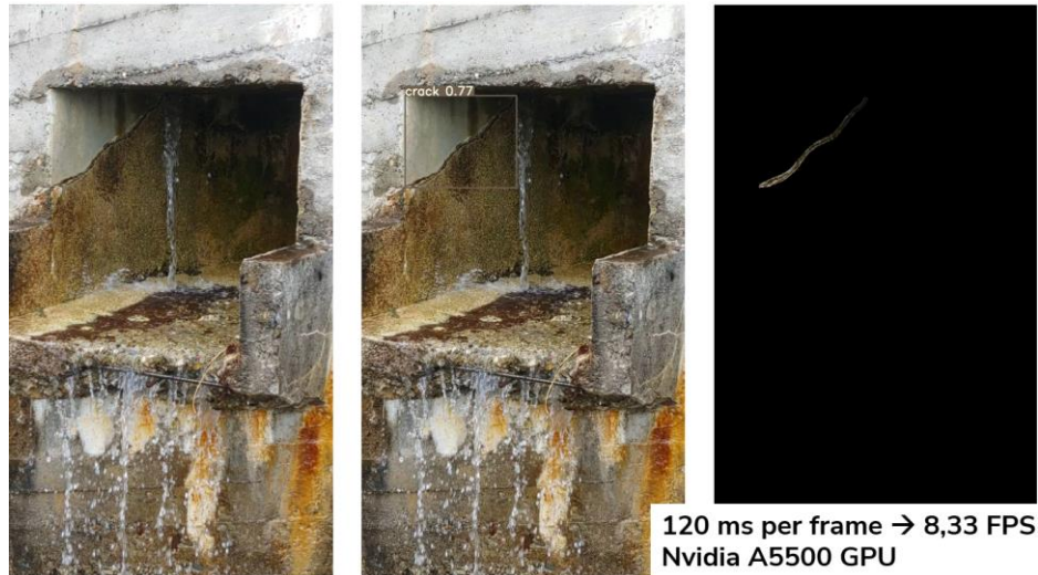
Figure 17: YOLOv8x-seg Crack detection and segmentation model inference examples on HDE premises.
